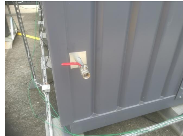
Ventilation and regulation
